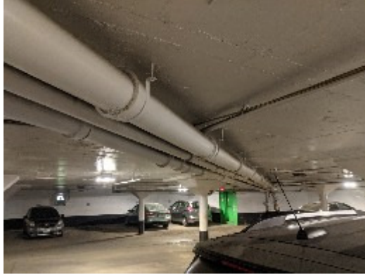
8. 30 Speers Rd, Hung SAN + STM laterals in parking garage
