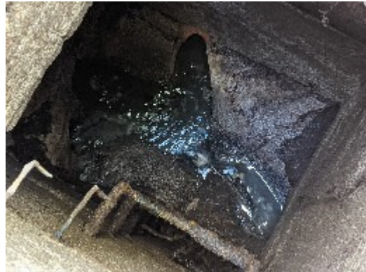
6. 80 Speers Road, MH SAN (Requires re-benching)
