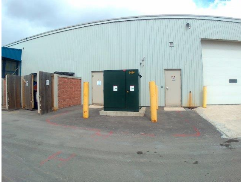
Photo 5 - View of pad mounted transformer to the rear of the Shoppers Drugmart (facing north).
