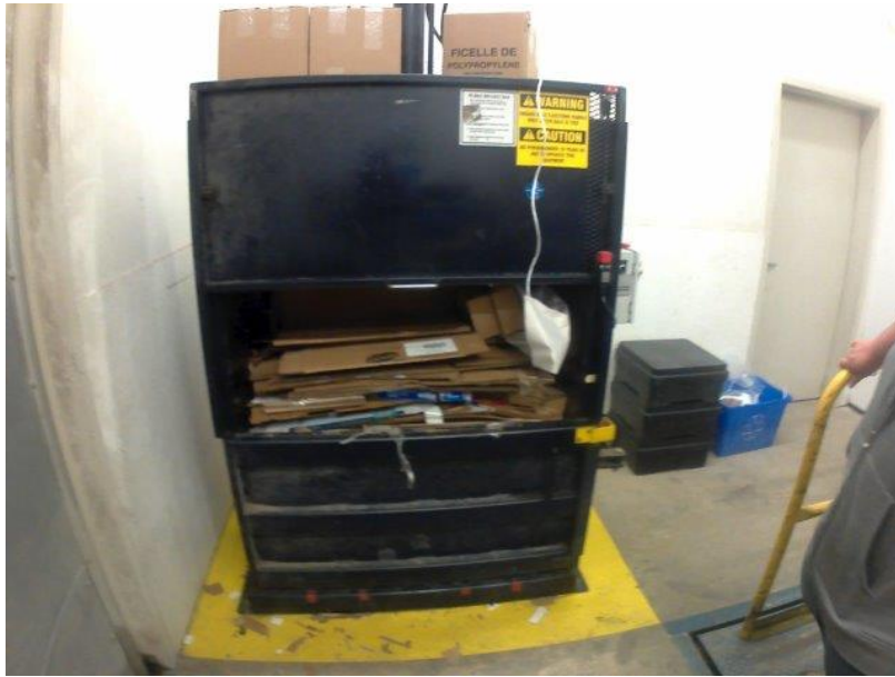
Photo 13 - View of the small, mechanical cardboard compactor within the warehouse area of the Shoppers Drugmart
