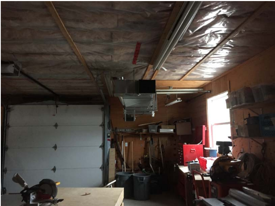
Natural gas furnace located inside the barn at the Phase One Property
