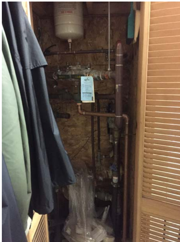
Hot water tank inside the main garden centre building
