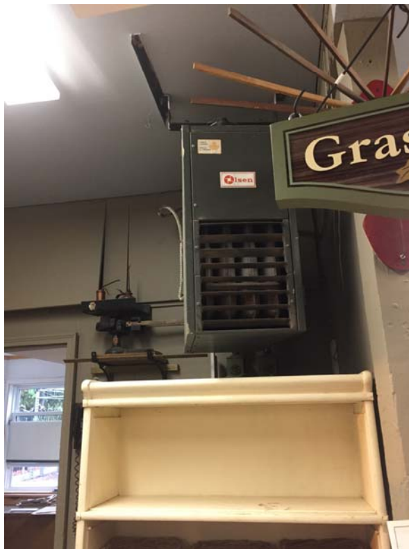
Natural gas furnace heating the main garden centre building
